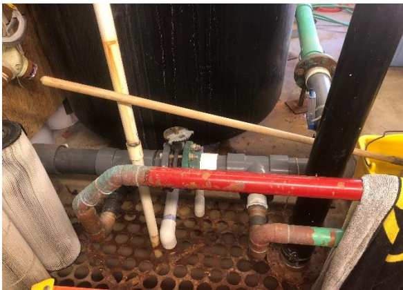
Photo #11: Backwash holding tank and pool.
