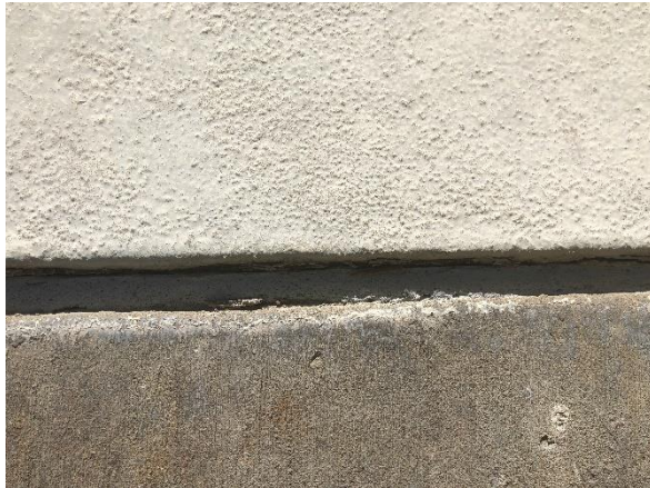
Photo #1: Joint between the pool liner and coping and pool deck.
