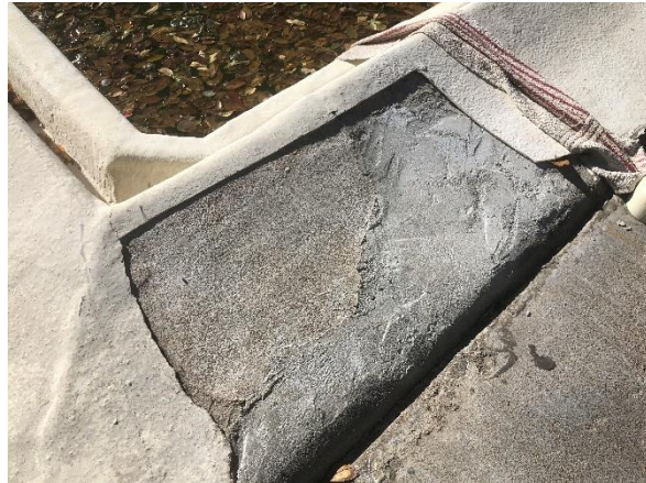
Photo #2: Pool liner failing.
