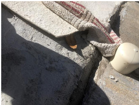
Photo #3: Further detail of pool liner failing. (Continuation of Photo #2)
