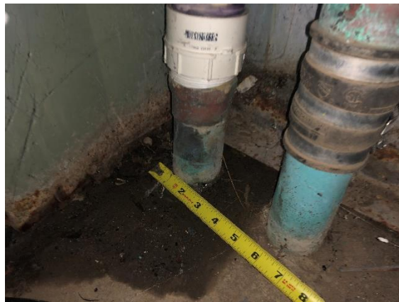
Photo #16: Suction piping
