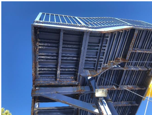
Photo #5: Corrosion at pool waterslide structure
