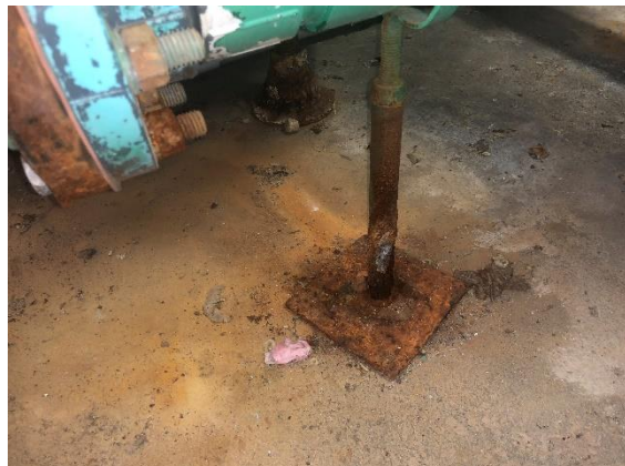
Photo #12: Corrosion of pool piping support.
