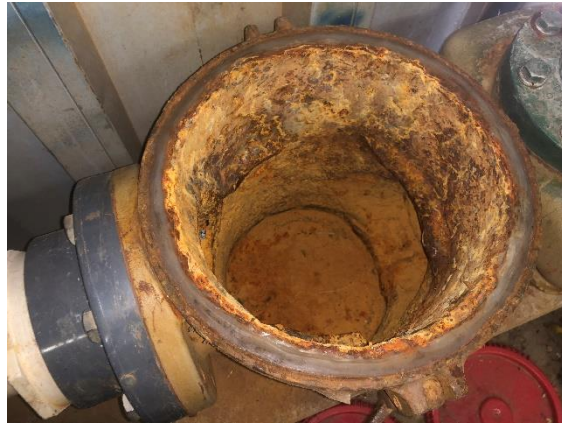
Photo #14: Corrosion at the pool strainer basket.
