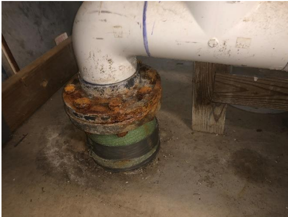
Photo #9: Transition from pool piping from mechanical room to below grade.
