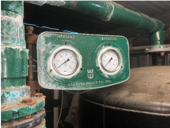
Photo #13: Filter Pressure Gauges
