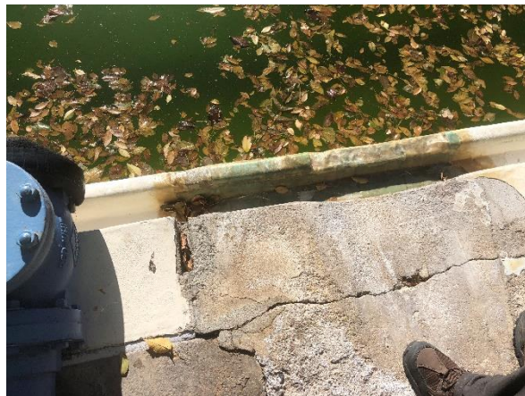
Photo #4: Location of pool slide entry. Location shows major wear of pool liner at slide entry point.
