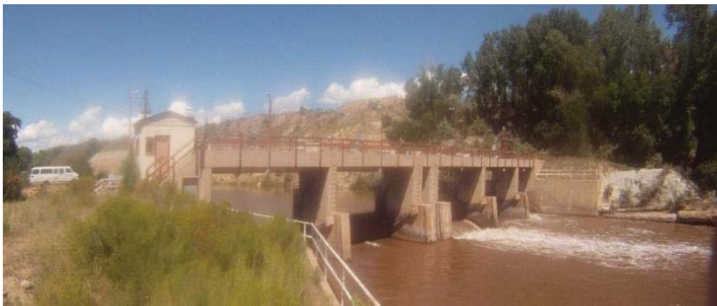
Minnequa Dam with its hazardous radial gates.
