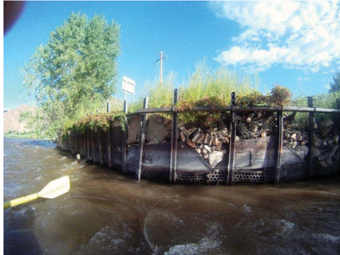
Existing intake for the power plant creates eyesore and safety issues.
